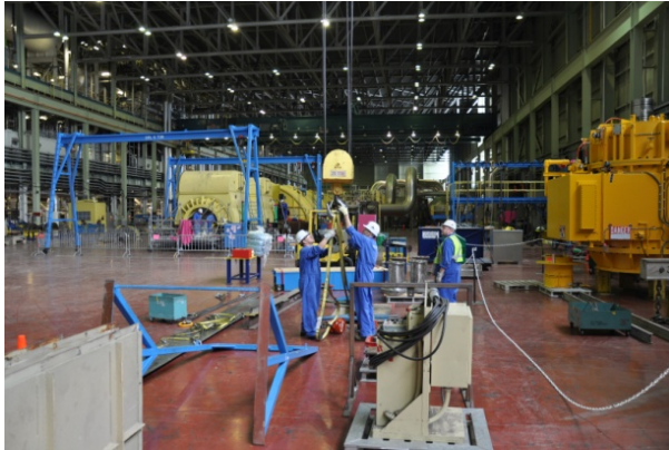
Bruce Power Unit 7 Outage Submitted by: Larry Alderdice
